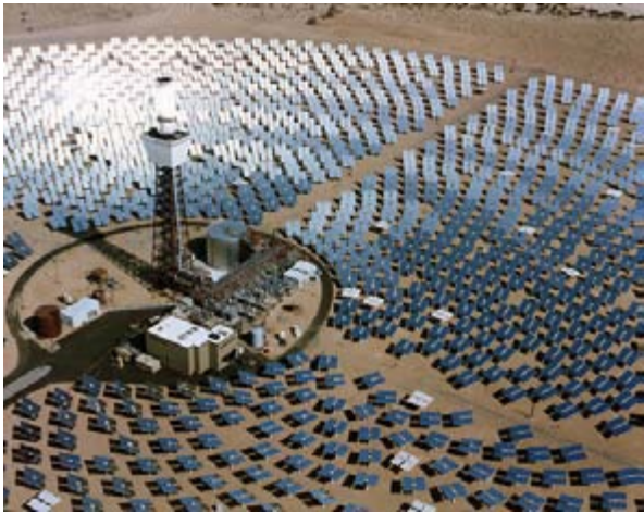
Figure A-6 10 MW Solar Two Power Tower System (Source: NREL)
